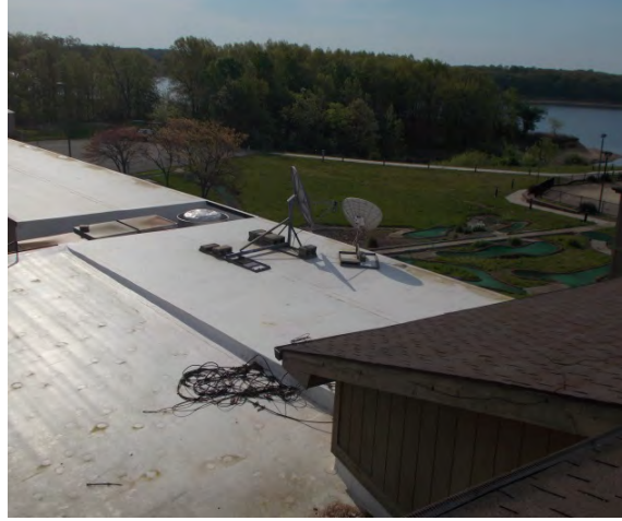
Figure 72- Existing Cable TV Dish Antennae
