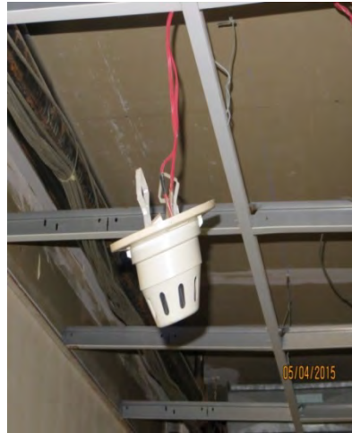
Figure 66 - Existing Smoke Detector In Public Corridor
