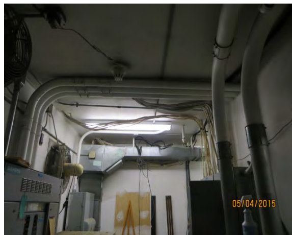
Figures 8 – Wires dangling in ceiling
