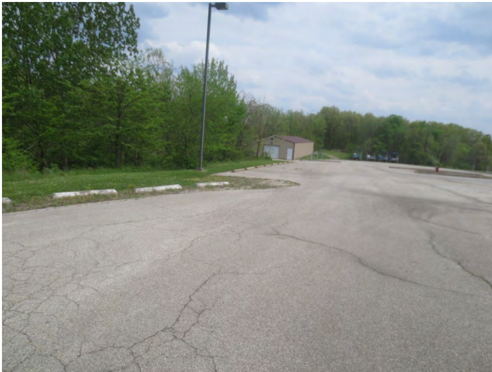
Typical pavement conditions south parking lot
