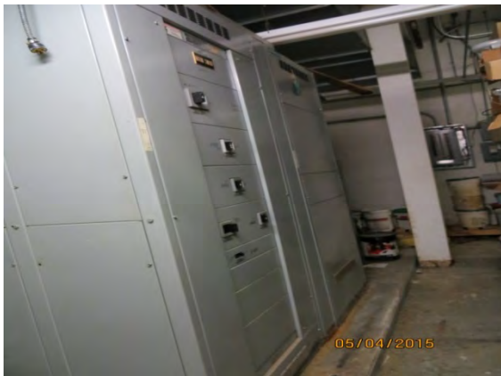
Figure 5 – 2500 amp, 277/480VAC main switchboard with corroded base
