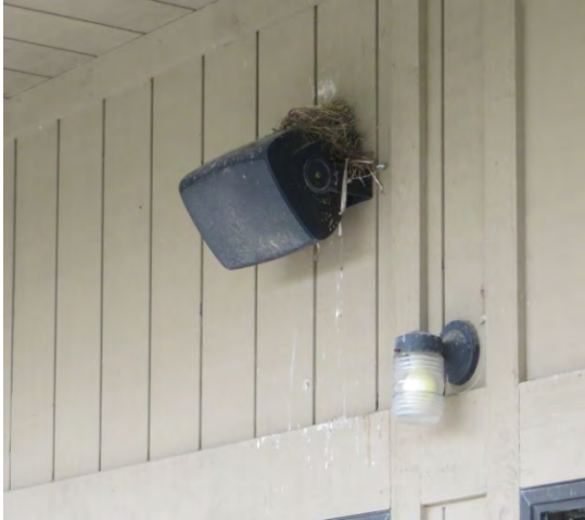
Figure 81 - Existing PA Speaker – Outdoor Swimming Pool Area
