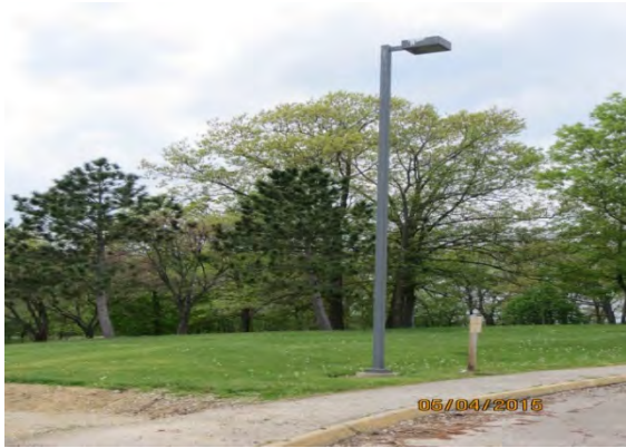
Figure 51 - Typical 30'-0" Pole Lighting
