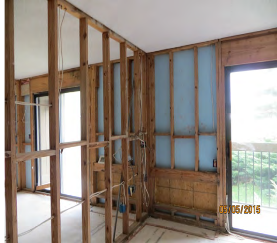
Figure 42 - Typical open wall for every hotel room – electrical outlets with non-metallic sheathed cable installation
