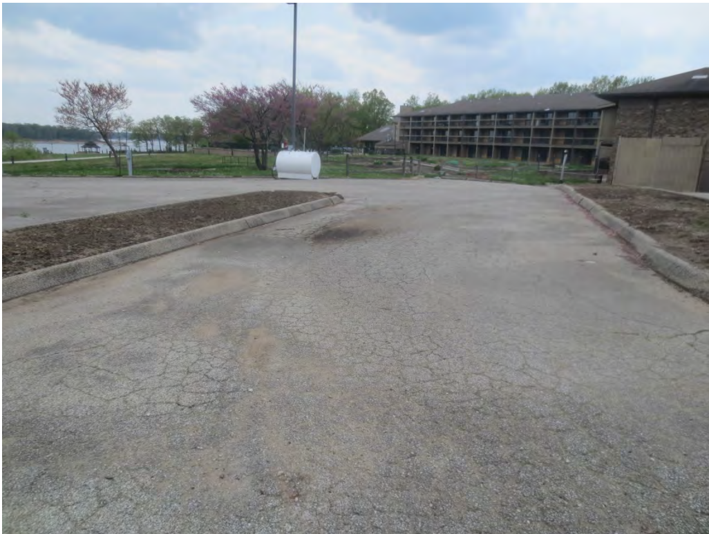
Alligator cracking northwest end of parking lot
