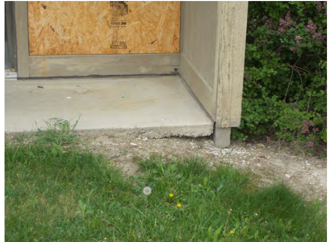
Figure 12 – Soil Erosion at Patio
