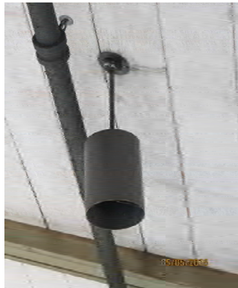
Figure 38 – Indoor swimming pool – pendant incandescent lighting fixtures
