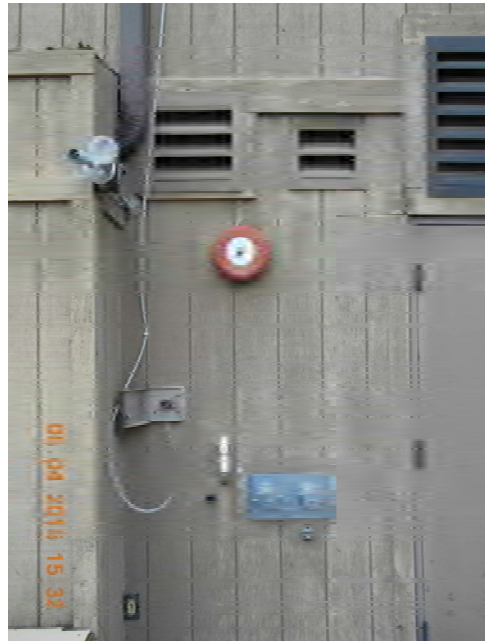
Figure 4 – Fire alarm bell
