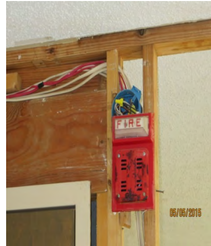
Figure 70 - Typical Audio Visual Alarm
