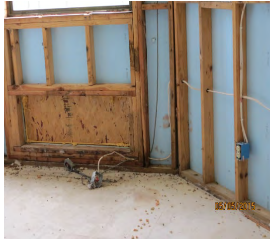
Figure 50 - Typical power outlet for Mechanical Unit
