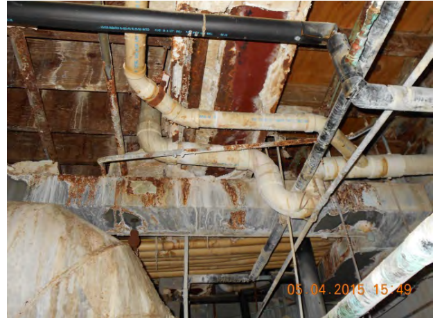
Figure 10 – Mechanical room ductwork corrosion
