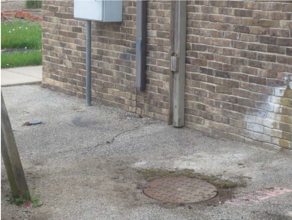
Roof drain discharging to pavement
