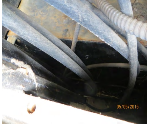
Figure 4 – Service feeders submerged in water
