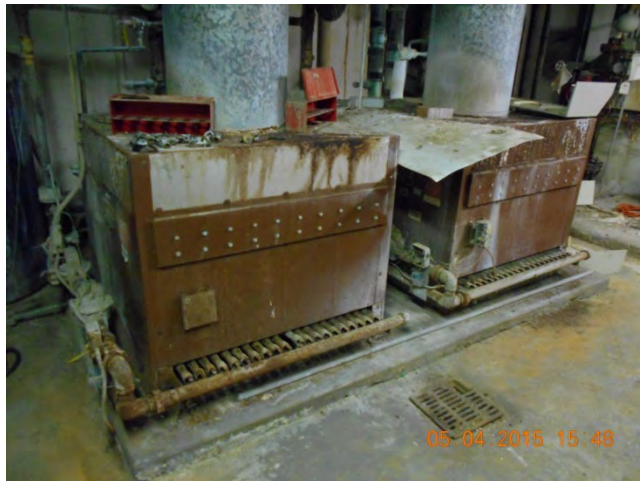
Figure 2 – Hot water boilers
