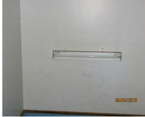
Figure 16 – Stairwell fluorescent lighting
