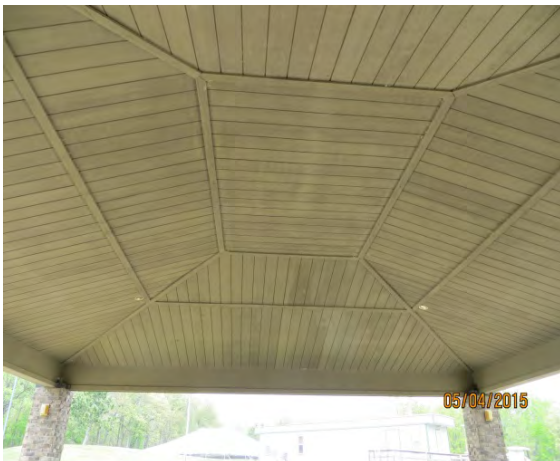
Figure 19 – Entry canopy lighting
