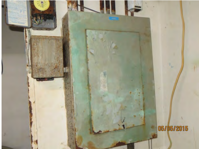
Figures 9 – Indoor swimming pool panelboard
