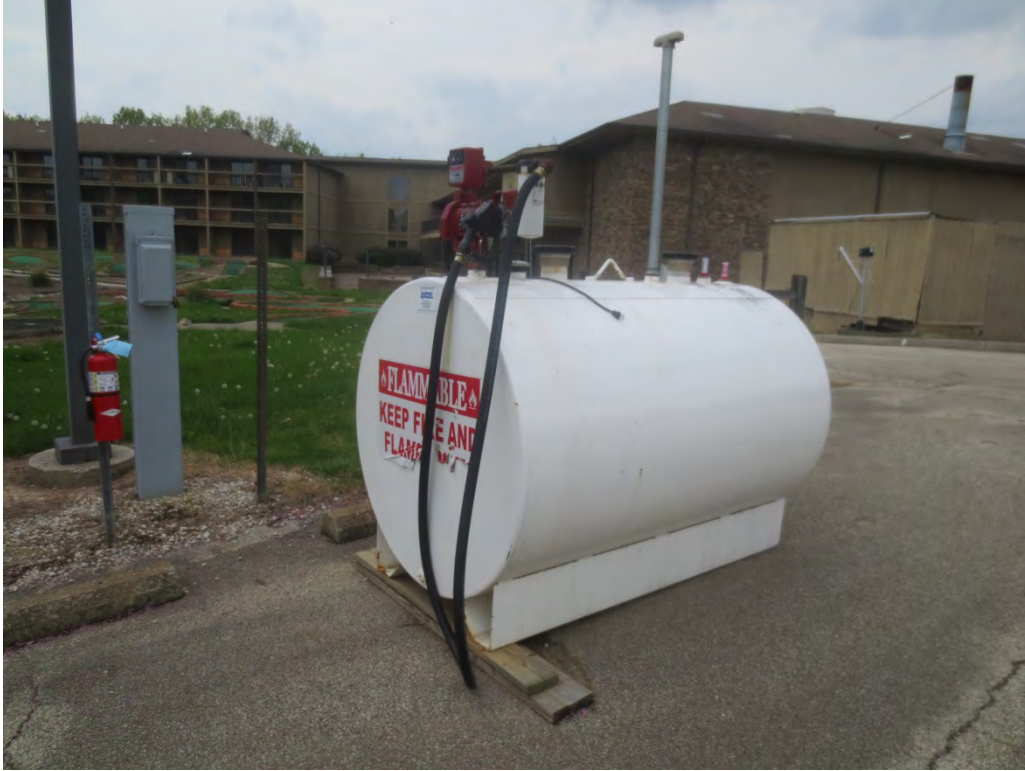
Unprotected fuel tank adjacent to mini-golf
