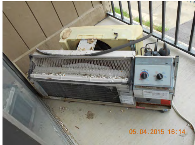
Figure 2 – Guestroom PTAC unit stored on balcony
