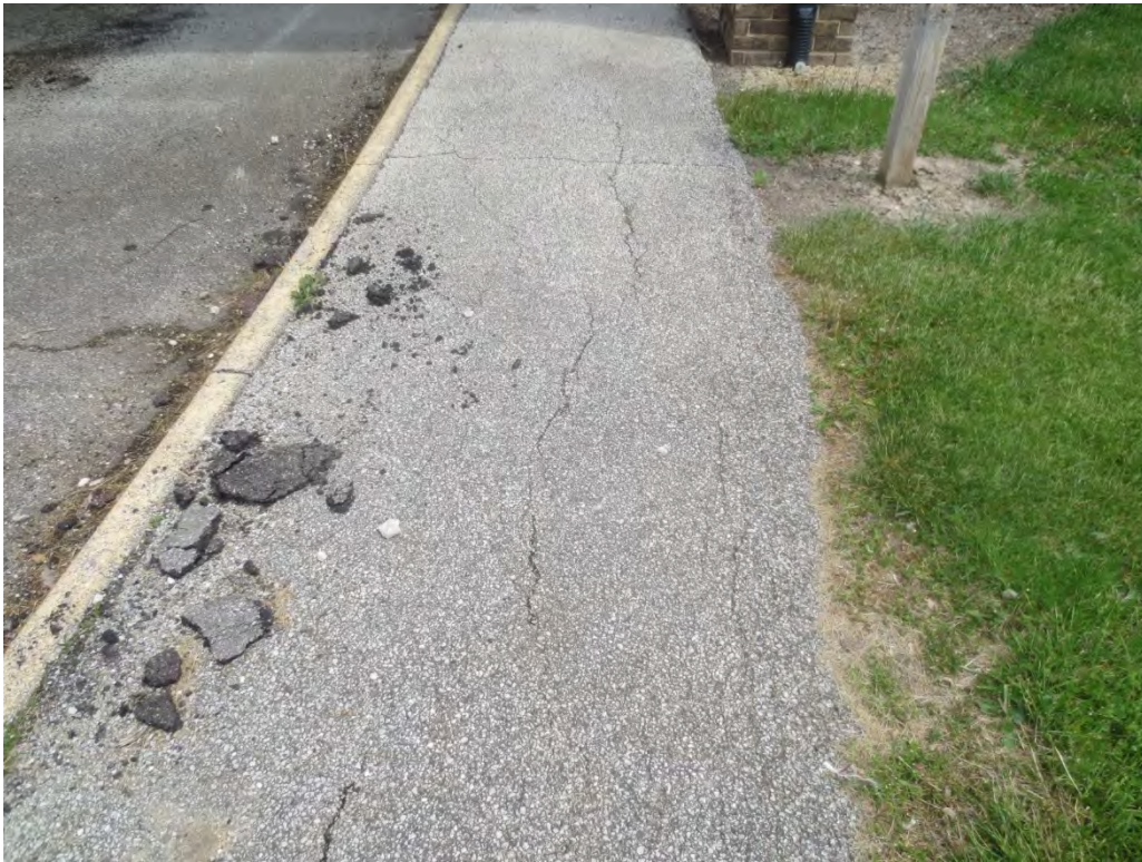
Typical asphalt sidewalk adjacent to roadways; minor cracking; debris is from roadway.
