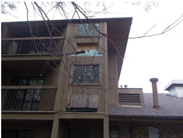
Figure 9 – Exposed A/C Openings in Wall
