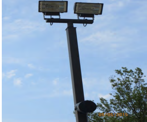
Figure 82 - Existing PA Speaker – Outdoor Swimming Pool Area
