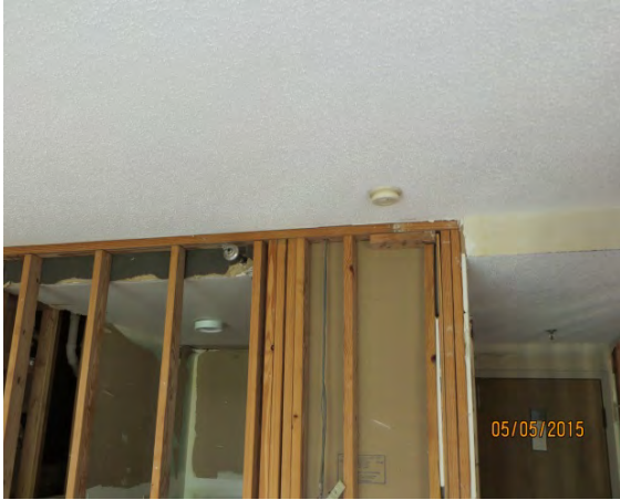
Figure 47 - Typical Ceiling Mounted Smoke Detector
