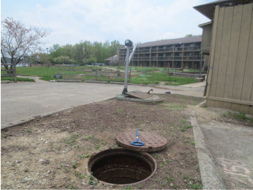
Pump and tank manholes
