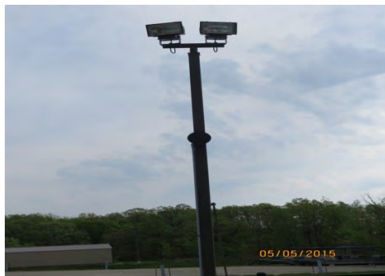
Figure 55 - Typical Outdoor Swimming Pool Flood Light HID Fixtures Building perimeter wall mounted fixtures need to be replaced (Figures 57 and 58).
