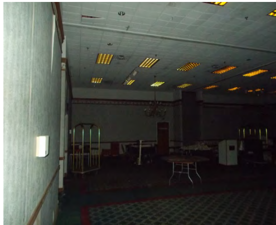
Figure 24 – Banquet areas: pendant and recessed lighting fixtures
