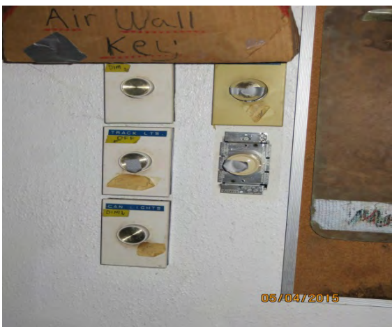
Figure 25 – Banquet area rotary dimmer switches
