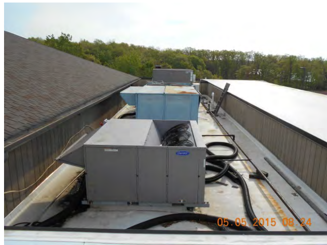
Figure 3 – Makeup air handling units in rooftop mechanical courtyard
