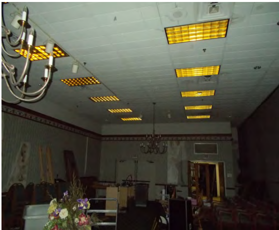
Figure 23 – Banquet areas: pendant and recessed lighting fixtures
