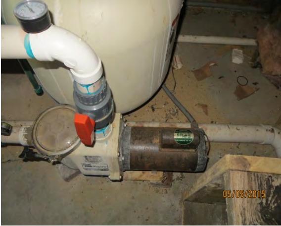
Figure 13 – Water pump purifier
