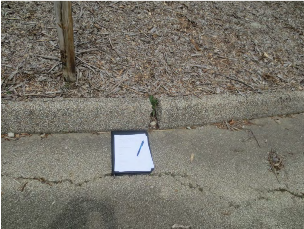
Asphalt curb cracks - typical
