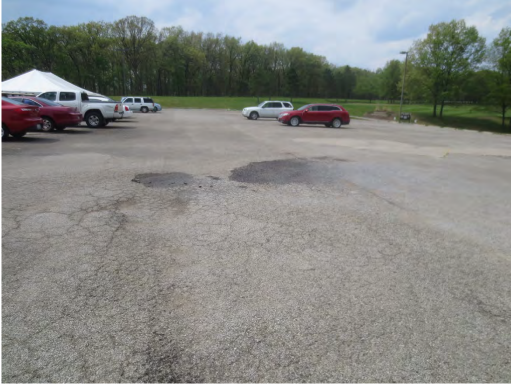
Evidence of localized ponding and pavement deterioration
