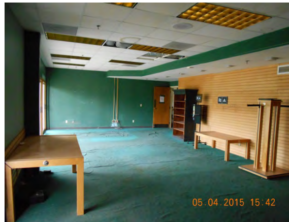
Figure 32 – Recreation area lighting
