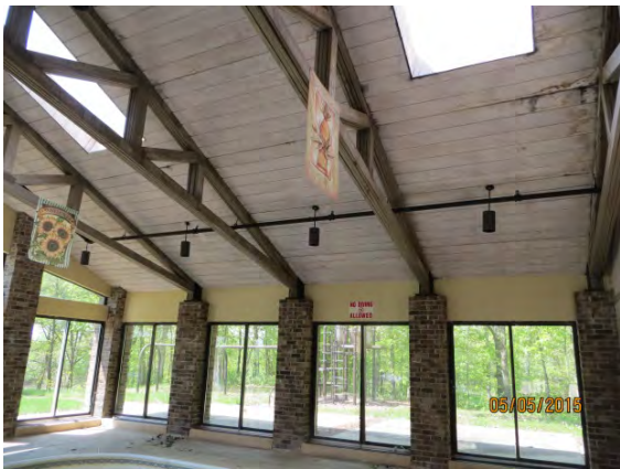
Figure 35 – Indoor swimming pool – pendant incandescent fixtures
