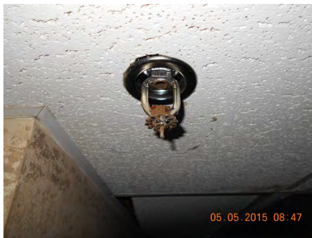
Figure 5 – Sprinkler head with fuse removed located in main hotel
