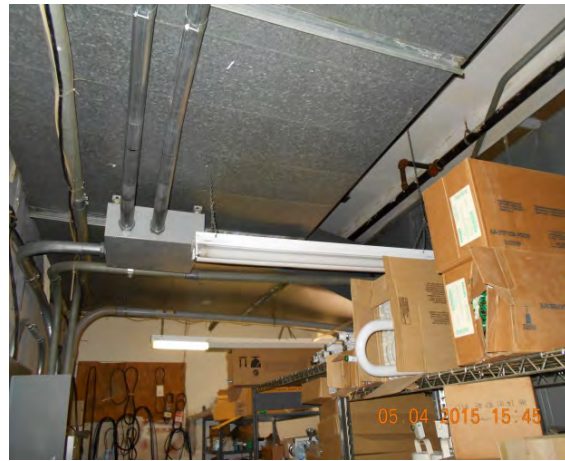
Figure 18 – Main switchboard room lighting
