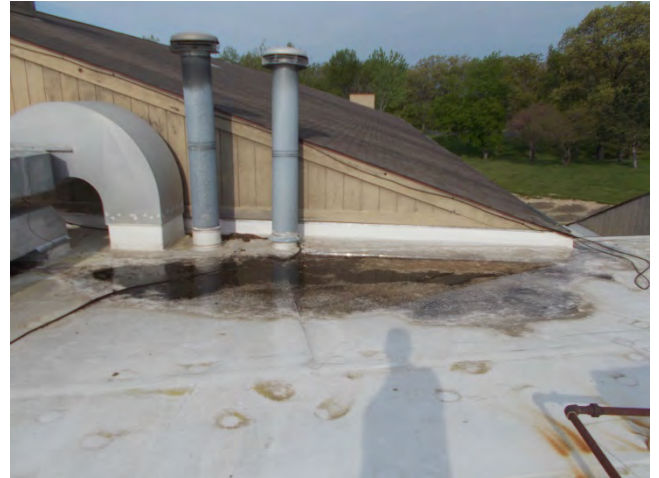
Figure 28 – Ponding at Flat Roof
