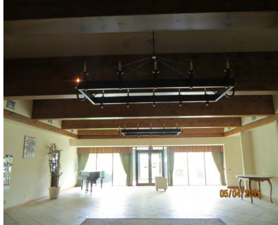
Figure 22 Main Lobby Lighting
