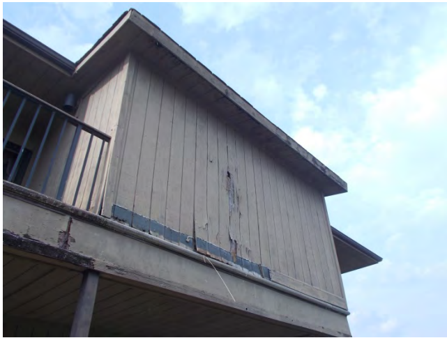
Figure 7 – Typical Wall Deterioration
