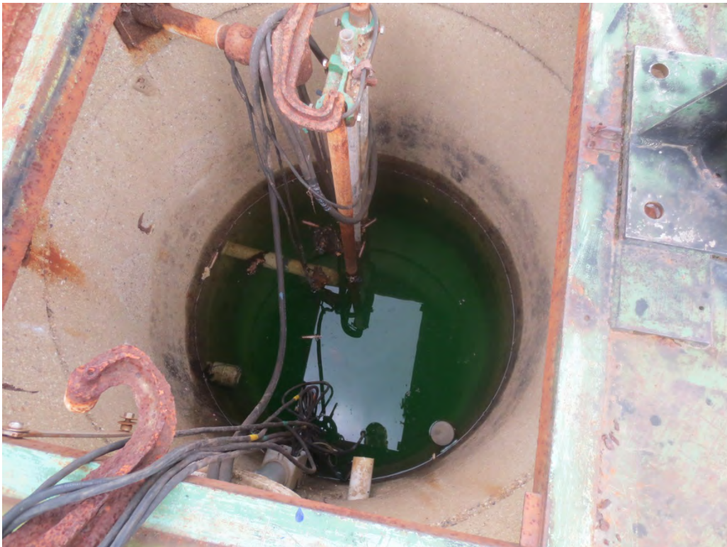
Pump station interior
