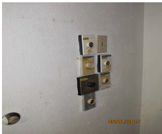
Figure 26 – Banquet area rotary dimmer switches
