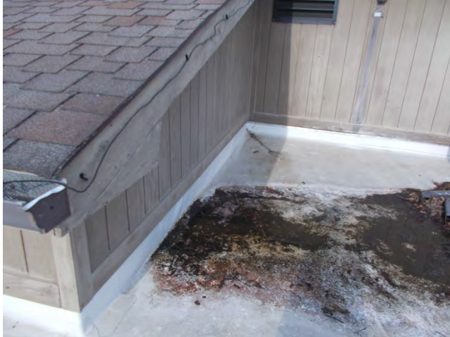
Figure 27 – Mold at Flat Roof
