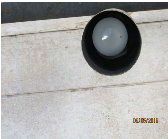
Figure 37 – Indoor swimming pool – pendant incandescent lighting fixtures
