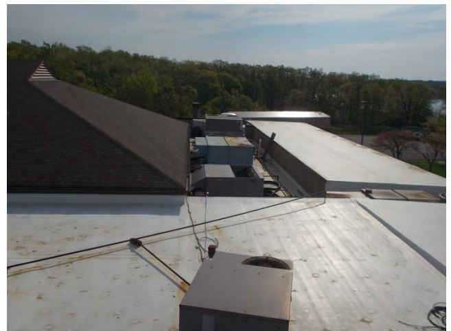
Figure 18 – Mechanical Equipment on Flat Roof
