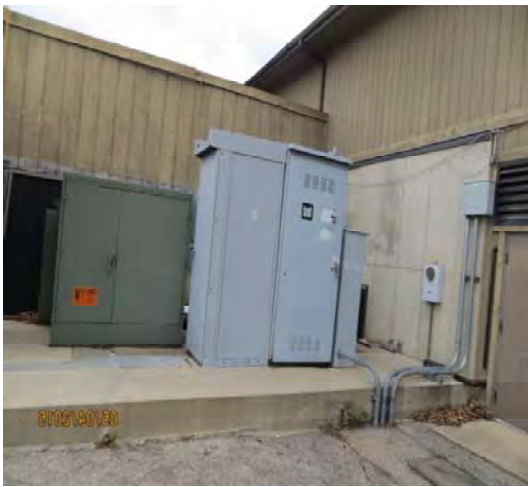
Figure 1 – Utility transformer and automatic transfer switch
