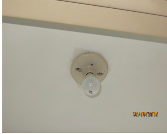
Figure 48 - Typical Suite Closet Light
