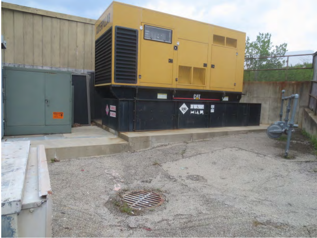
Back-up generator with belly tank. Note catch basin.
