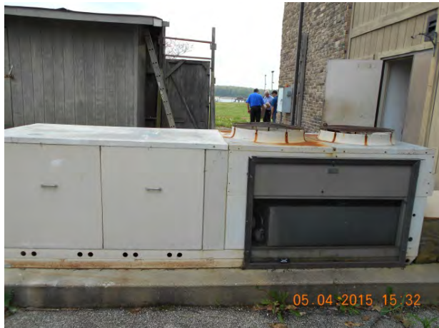
Figure 7 – Walk-in cooler condensing unit
