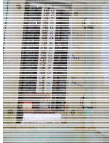
Figure 10 – Indoor swimming pool panelboard interior
