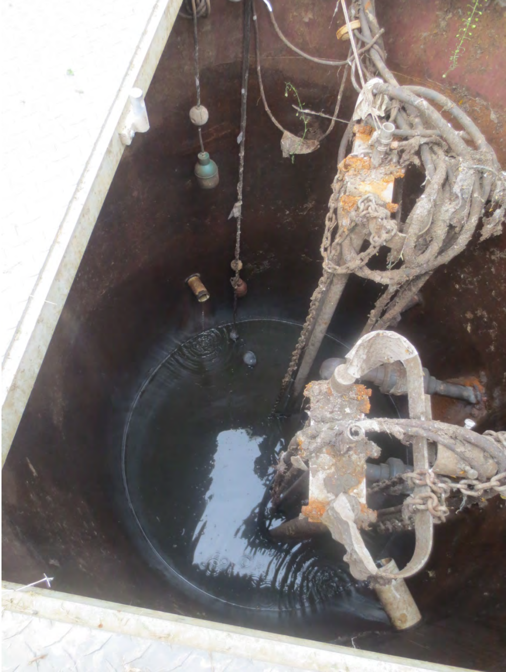
Berry Pond Pump Station
