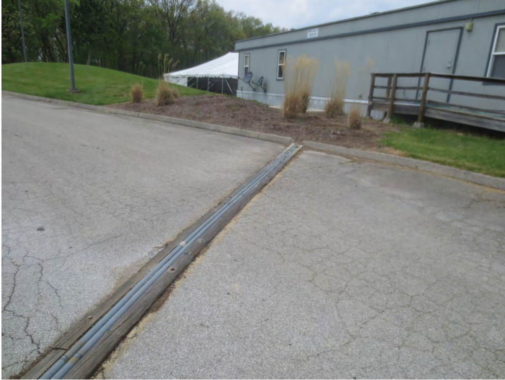
Water line leading to the temporary Pro Shop Trailer
