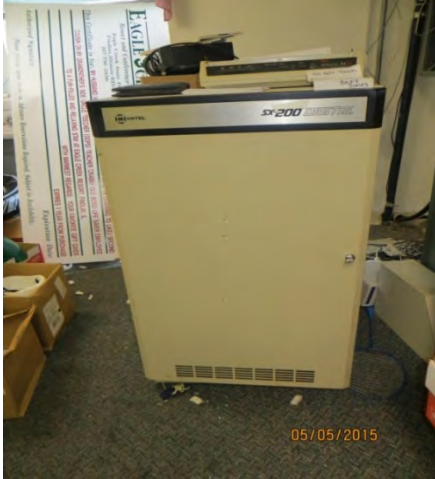
Figure 60 - Existing Main Telephone Server (SX 200 Digital)
