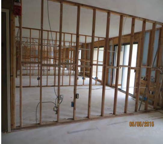
Figure 41 - Typical open wall for every hotel room – electrical outlets with non-metallic sheathed cable installation
