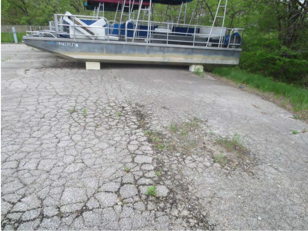
Significant pavement deterioration south end of parking lot
