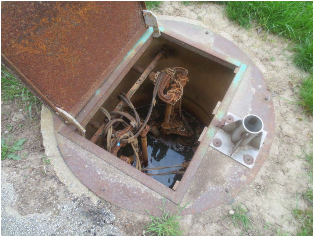
Eagle's Landing Sanitary Sewer Pump Station
