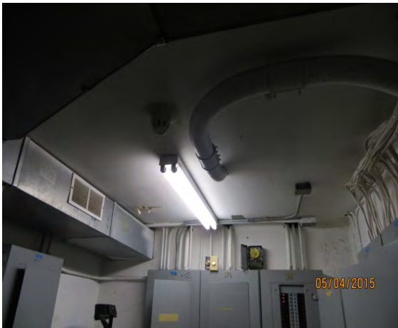
Figure 17 – Typical electrical room lighting
