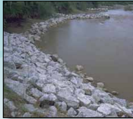
Rock was placed along streams in the Spoon River Watershed to stabilize the banks from eroding.
