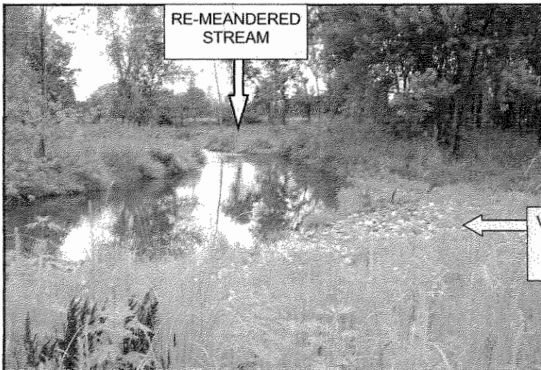
Photo: Phase 1 diversion berm to divert stream flow through the meandering channel (direction of flow is from foreground to background in photo).
