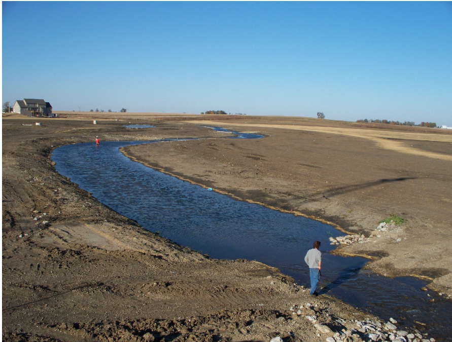
Figure 17. This is an overview of the completed construction work on the west branch of Phase 1. One of the constructed wetlands is also visible in the background to the left of the stream.
