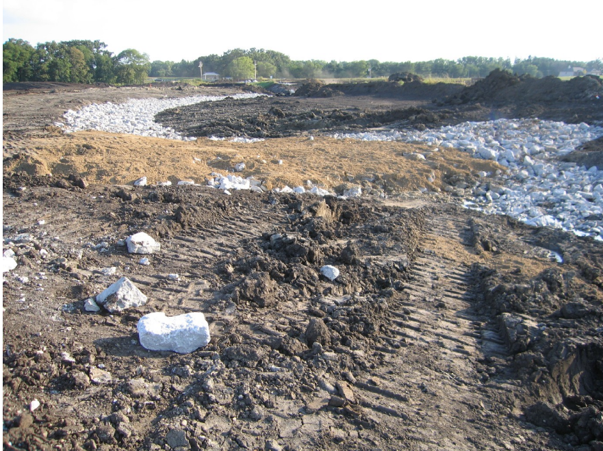
Figure 14. This photograph shows a view of the newly constructed stream channel prior to diversion of water. The armored banks can be seen in the background with one of the Newbury weirs in the foreground. The Newbury weirs were topped with a CA6 sand and gravel mix to seal the rock crevices and provide a more natural substrate type for ecological benefits.
