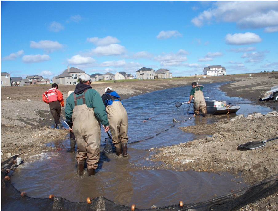
Figure 27. A post-restoration sampling event on the downstream treatment site on the west branch (EIEM-01). This sample was conducted just days following completion of the stream channel construction work in 2008. Note the use of the electric seine and blocknets to isolate the sampling reach.
