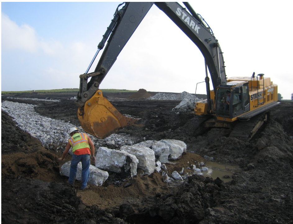
Figure 12. Peak stones were placed to secure the placement and integrity of the Newbury weirs.
