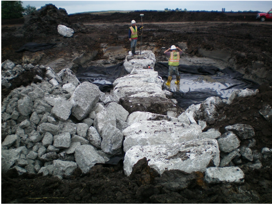
Figure 13. The peak stones set the height of the Newbury weirs. This was checked carefully with GPS equipment, as riffle height is critical to the function of the weir.
