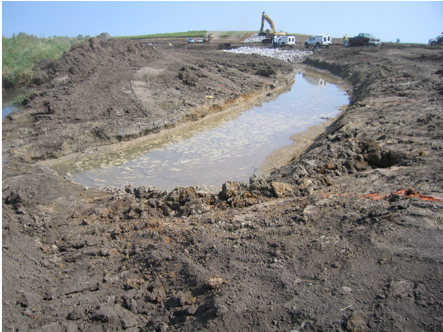
Figure 9. The new channel was constructed “in-the-dry” adjacent to the existing channel (seen in the upper left hand corner of this photo). Water within the excavation is groundwater seepage, which is a contributing factor to the high quality of this stream system.
