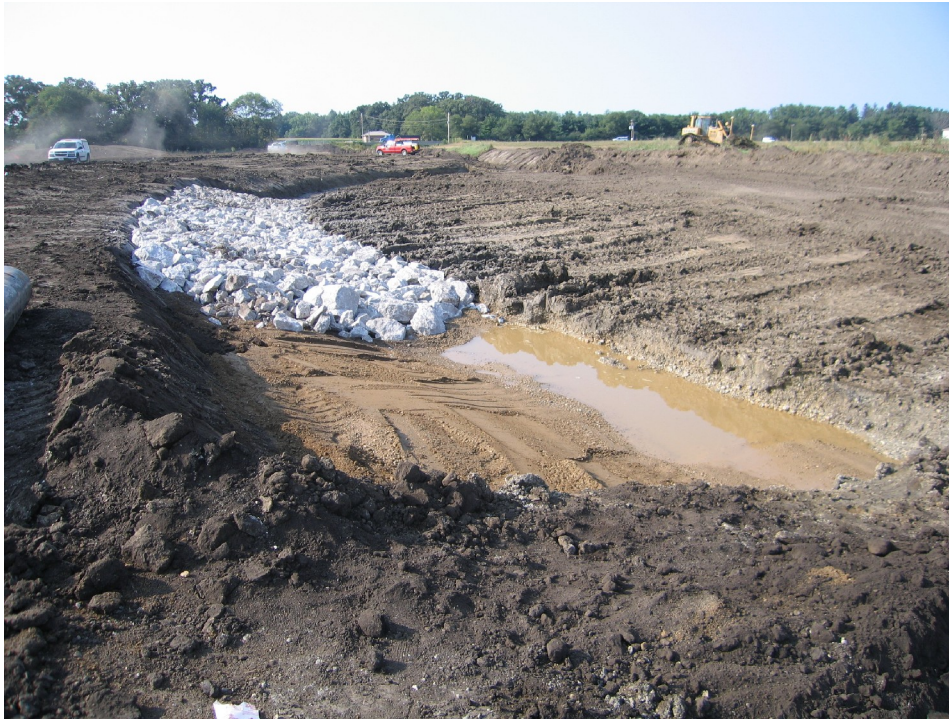
Figure 11. Outside bends were heavily armored with rip rap to maintain the path and form of the new channel.
