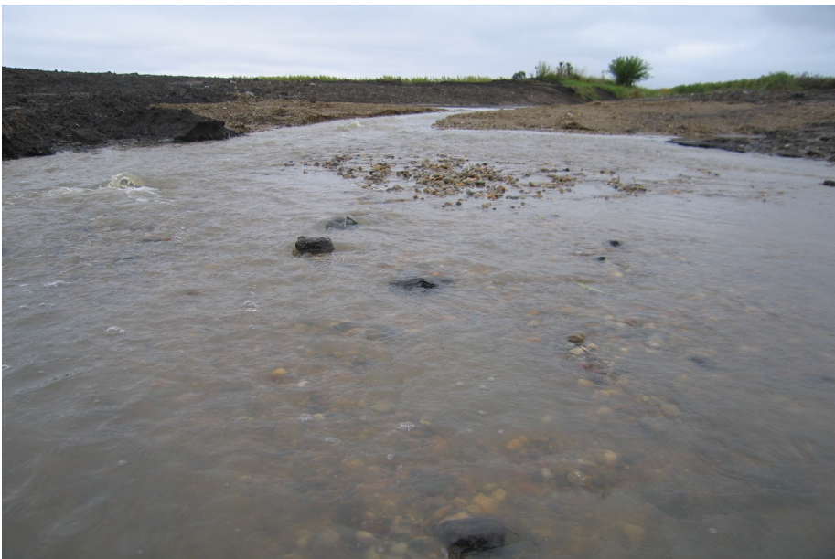
Figure 16. This view is a close-up of one of the Newbury weirs, showing how the CA6 mix allows the weir to closely mimic a natural riffle just days after construction.
