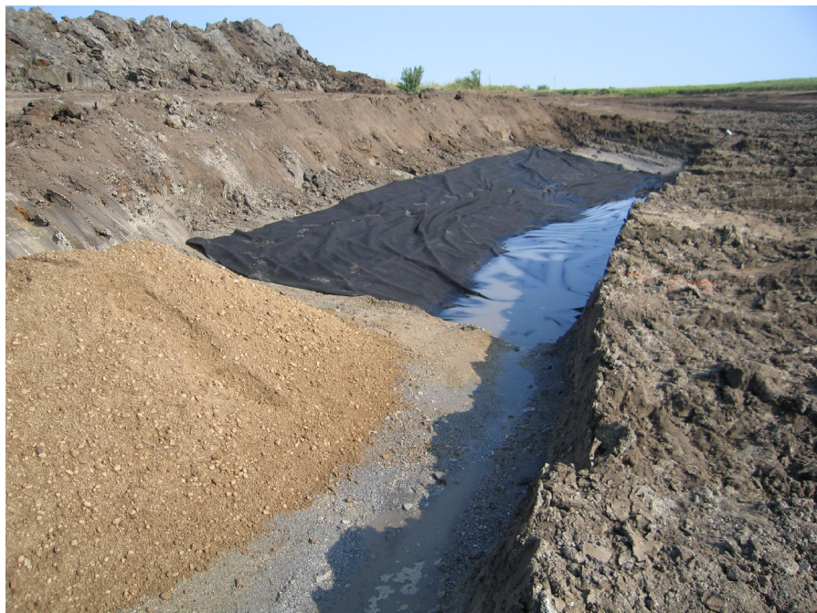
Figure 10. Fabric was laid in the base of the excavated new channel and covered with a sand and gravel mix.
