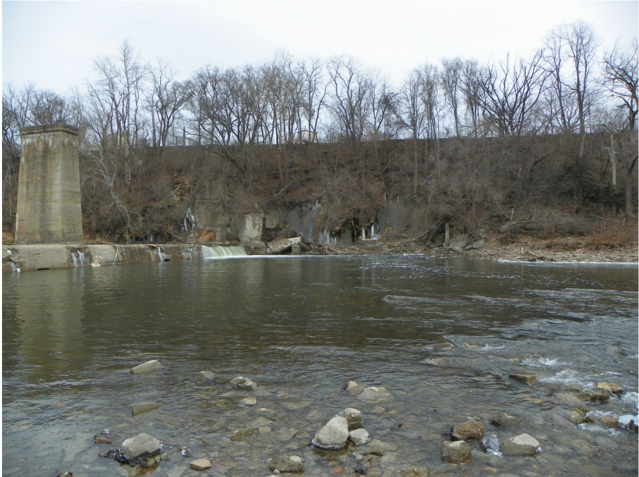
Figure 5 – Danville Dam on the Vermilion River. Photo taken on January 2, 2014 showing continued structure failure.
