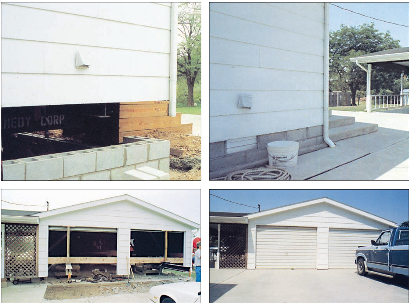
Figure 10 The coal company took measures to protect this home in advance of subsidence. Structures were raised from the foundations and kept level during subsidence. Foundations were restored and structures lowered onto them after damaging ground movements ceased.
