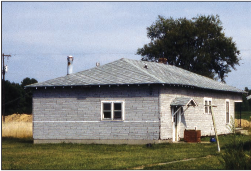
Figure 11 This unoccupied structure located above the centerline of a longwall panel was subsided 4.5 feet. The white line represents the level of the original ground surface.
