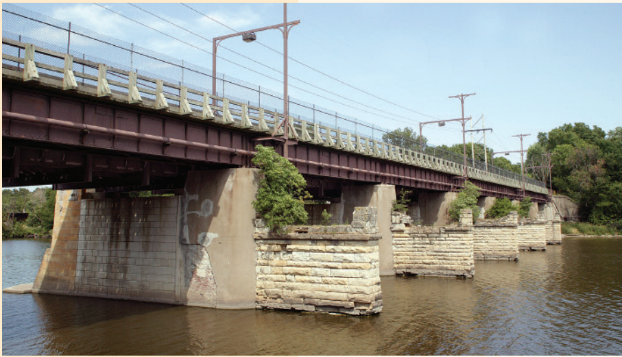
Where water once flowed through the 464-foot Fox River aqueduct at Ottawa, bikers and hikers now traverse.
