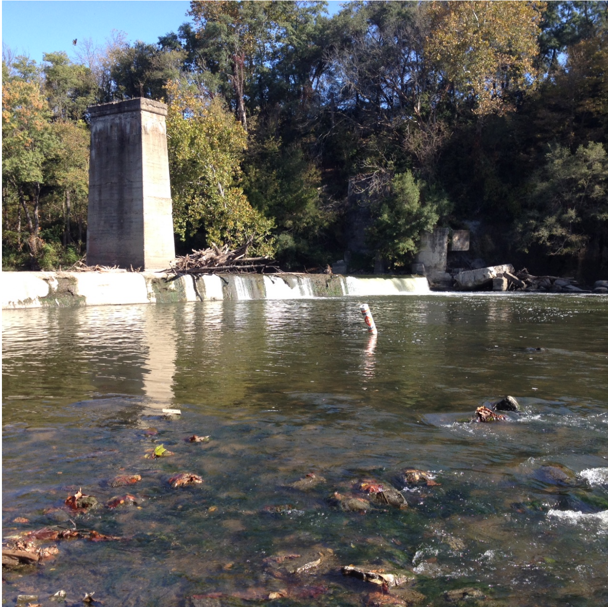
Figure 7 – Danville Dam photo from October 14, 2015 showing seepage along the face of the dam during low flow conditions.
