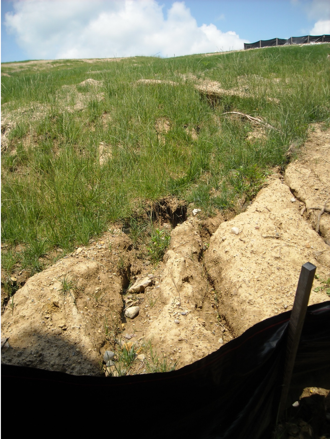
Figure 3b. Erosion impacted area on the southern flank of the cap.
