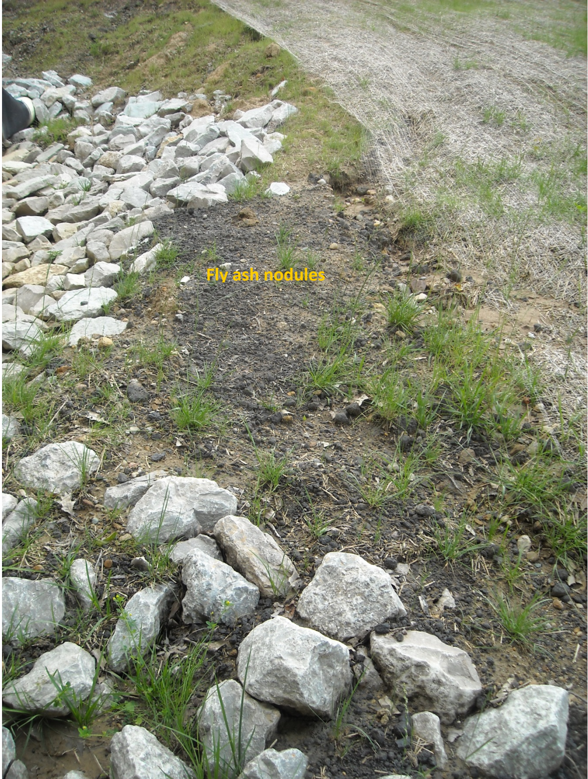
Figure 3c. Erosion impacted area on the southern flank of the cap with fly ash nodules clearly visible.
