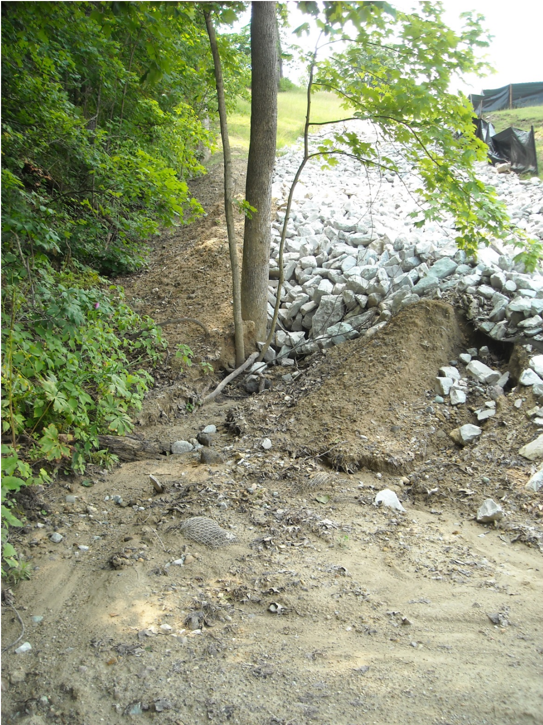
Figure 3a. Erosion impacted area on the SE side of the cap.
