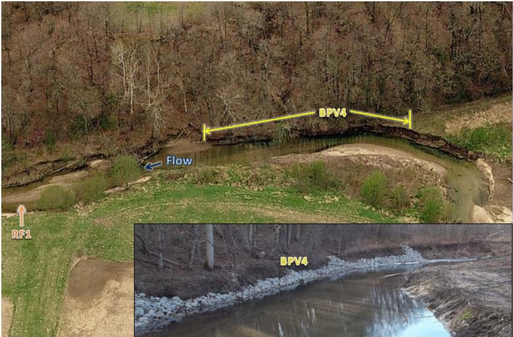
Figure 8. Condition of bank before peak stone installation at BPV4 (top-looking south) and after installation (bottom right-looking upstream).
