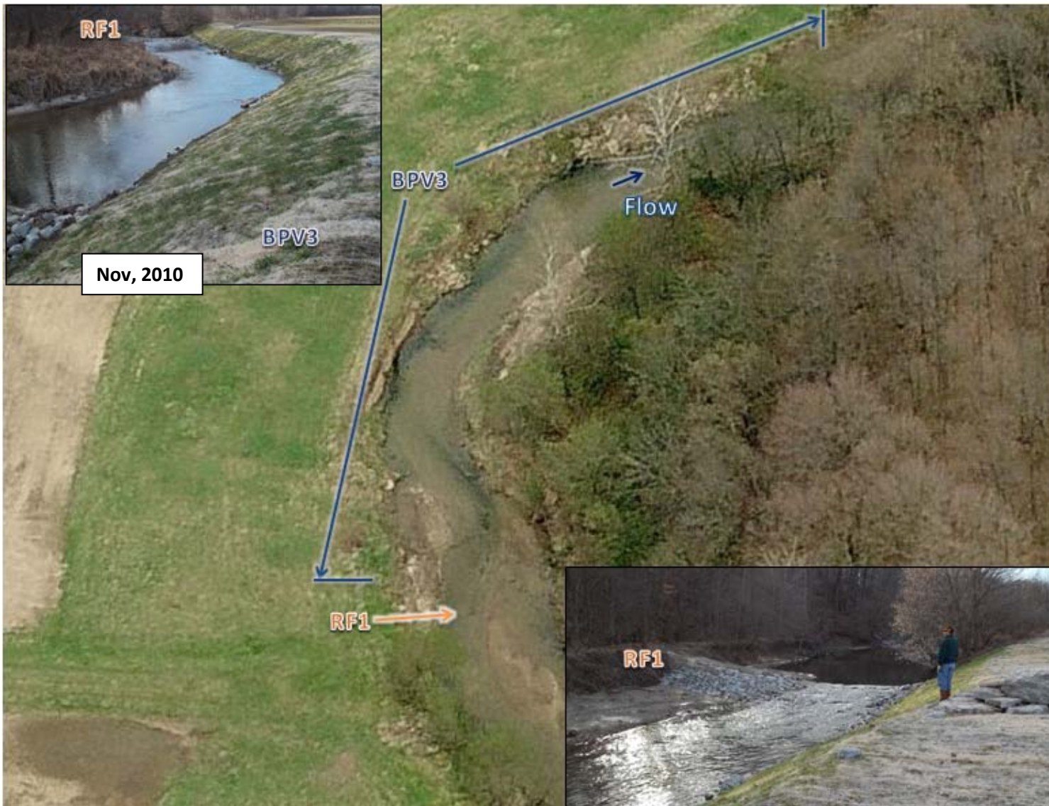
Figure 4. Condition of banks and stream before riprap sloped bank and riffle installation at BPV3 and RF1 (center-looking east) and after installation (top left and bottom right-both looking upstream).
