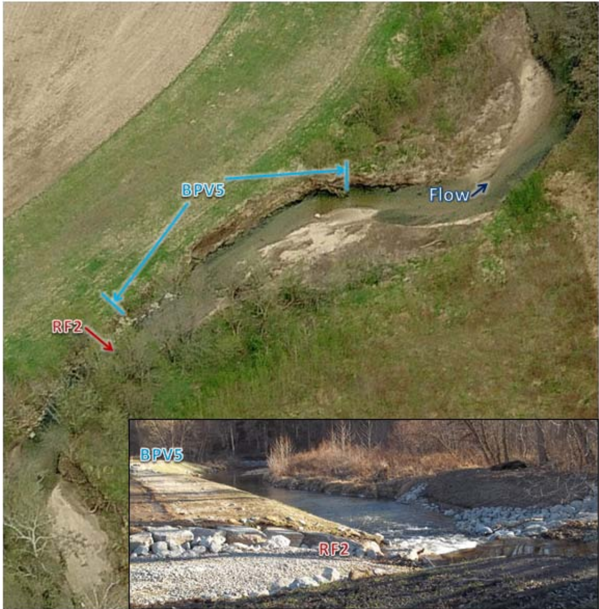
Figure 10. Condition of banks and stream before riprap sloped bank and riffle installation at BPV5 and RF2 (top-looking east) and after installation (bottom right-looking downstream).
