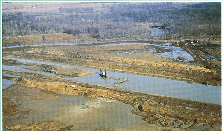
A dredge digs a nine-foot navigation channel through the Kaskaskia River bottom in the early 1970s. The dredge slurried water with sediment and soil and pumped it into large settling ponds. The project straightened the river by cutting through bends, significantly shortening it.
