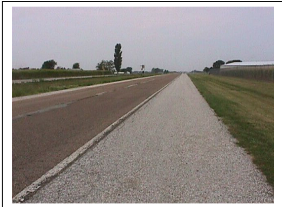
Figure 5- Existing Paved Shoulder on HWY 104 Should Be Striped As a Bike Lane
