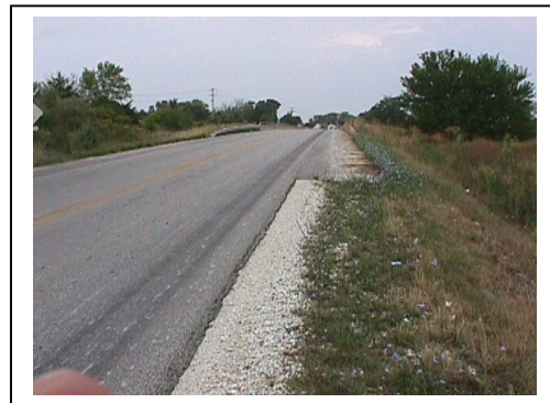
Figure 4- Paved Shoulder Needed along State Street
