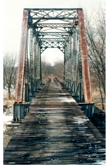
A piece of Heartland Pathways: Truss Bridge Across Salt Creek Near Weldon Springs (Piatt County) Photo courtesy of http://www.prairienet.org/heartland-pathways/heartlnd.htm
