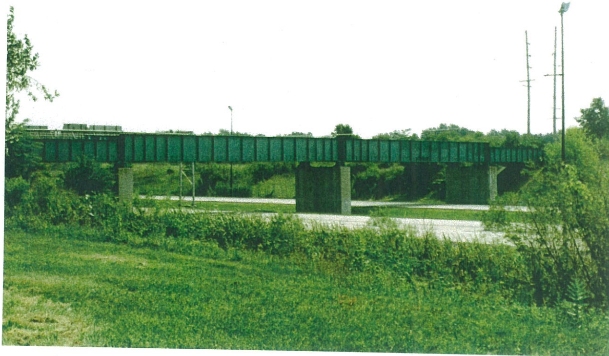
Abandoned rail lines, like this bridge crossing I-72 south of Forsyth, may provide useful bikeway connections.
