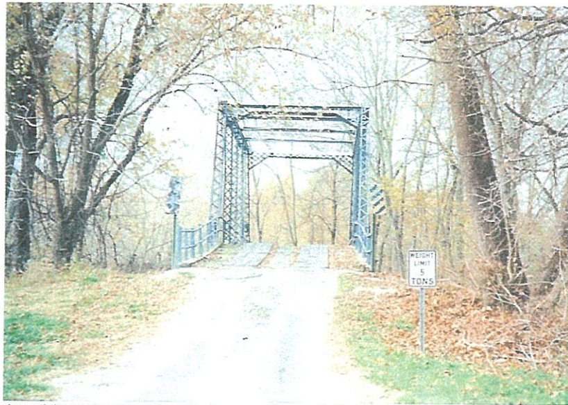
A view of the Valley Road truss bridge over Macoupin Creek south of Beaver Dam State Park.
