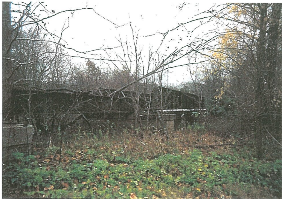
One of two remaining structures in Macoupin County is the former truss bridge carrying ITRR over Cahokia Creek north of Staunton.
