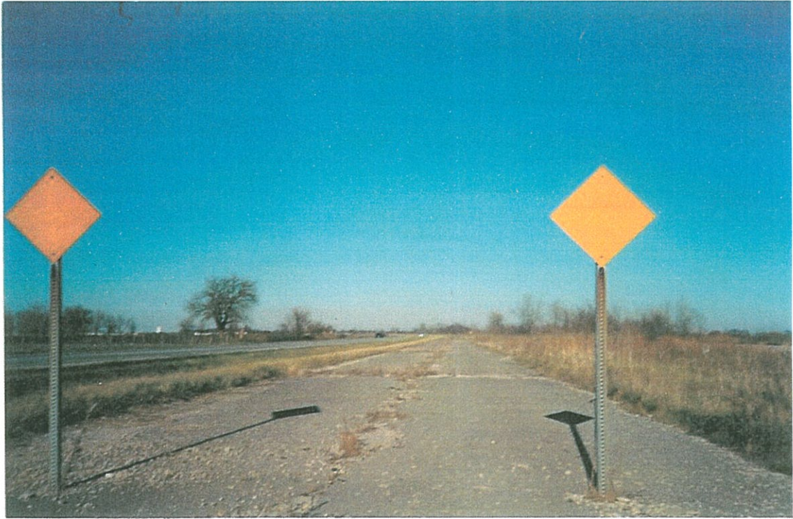
A typical section of the old Route 66 northbound lanes closed to thru traffic north of Mt. Olive.
