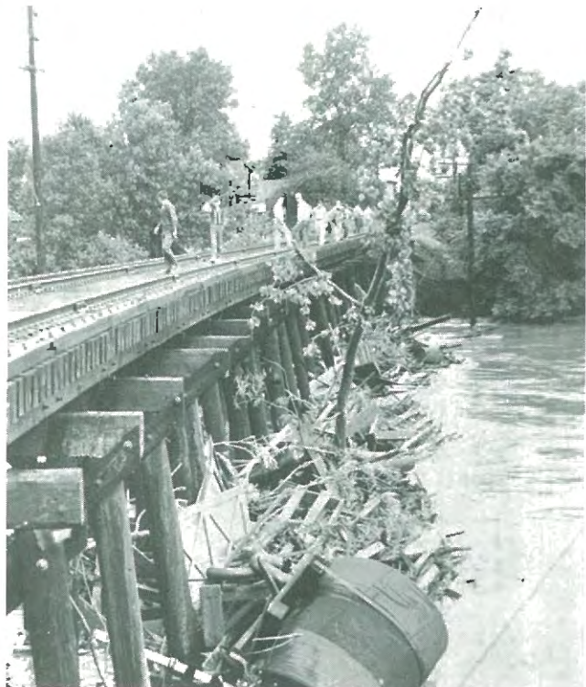
Debris piled against the Southern Railway trestle across Richland Creek in Belleville during the June 1957 flood.
